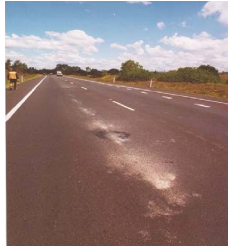
Bruce Highway near Gympie showing "pumping" of fines
